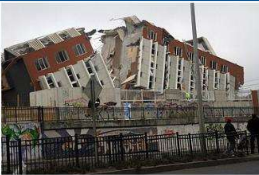
Damage sustained by a building in Concepción, located around 100 kilometres south of the epicenter.
