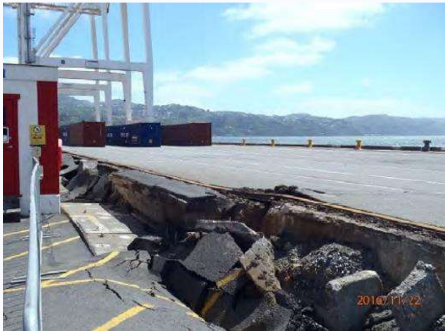
2016 M7.8 Earthquake, Wellington Centreport
